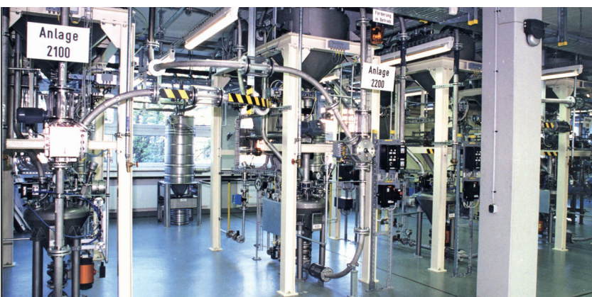
Feeding vessel conveying for chemical production
