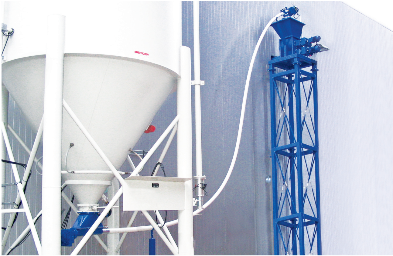
Silo discharge and metering screws - feed
