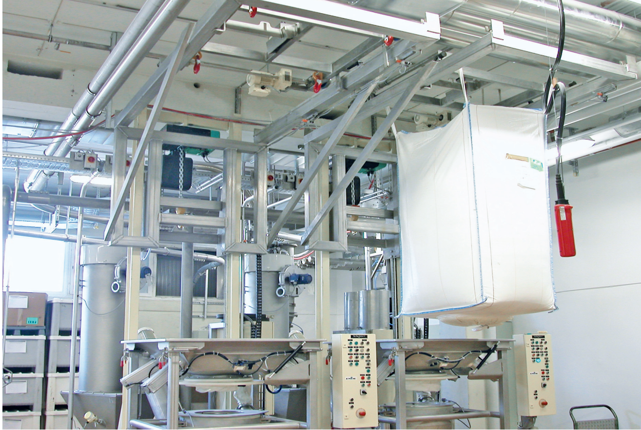
11 Big Bag emptying station with movable carrying frame
