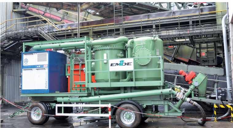
Mobile vacuum cleaning system in operation; antisurge protection resisting 10 bar excess pressure
