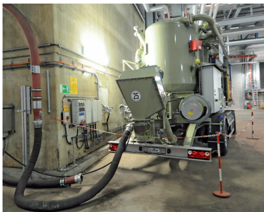
Flexible hose connection with pipe net
