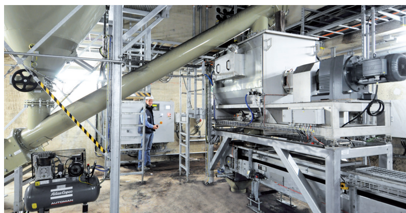
Moistening station with ribbon blender
