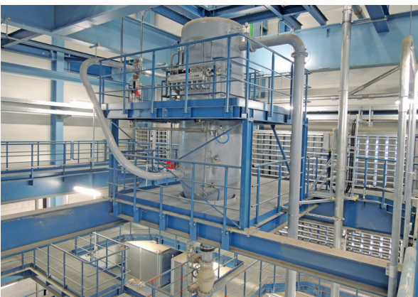
Vacuum cleaning system in power station
