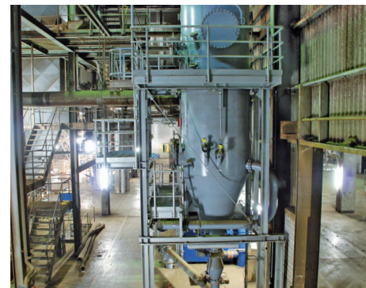
Filter separator with discharge sluices
