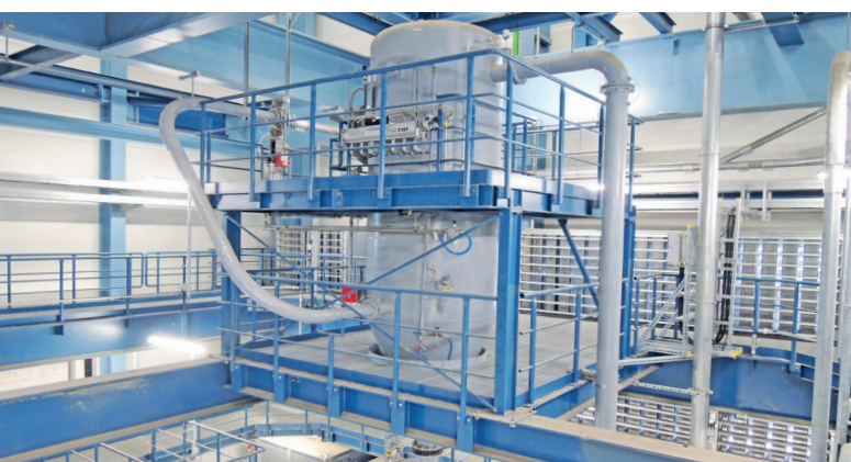
Vacuum cleaning system in power station
