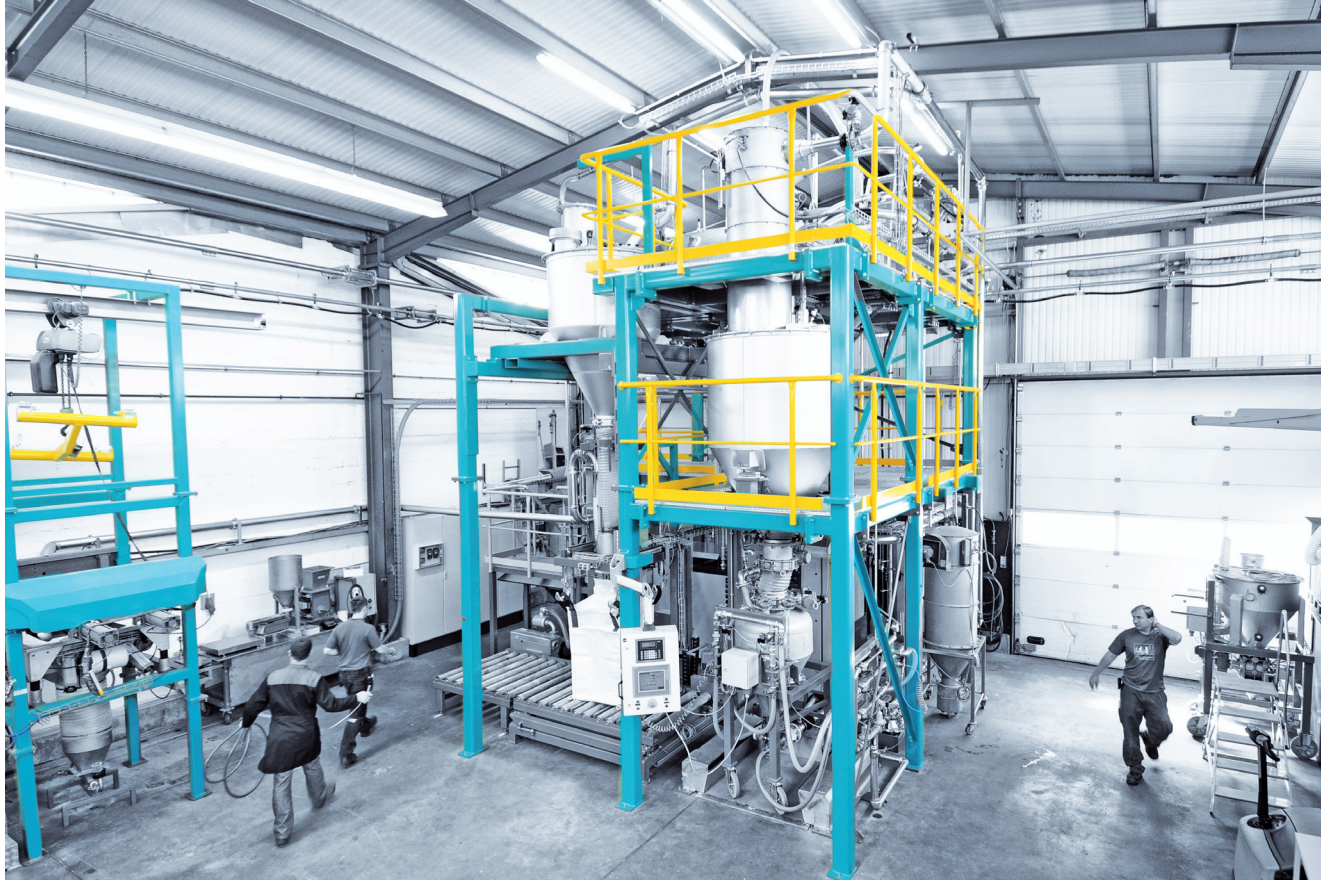
Technical centre equipment for pressure and vacuum conveying
