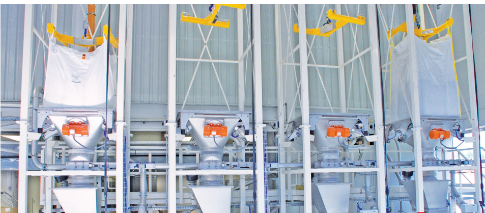
Big Bag emptying stations for the charging of differential metering scales
