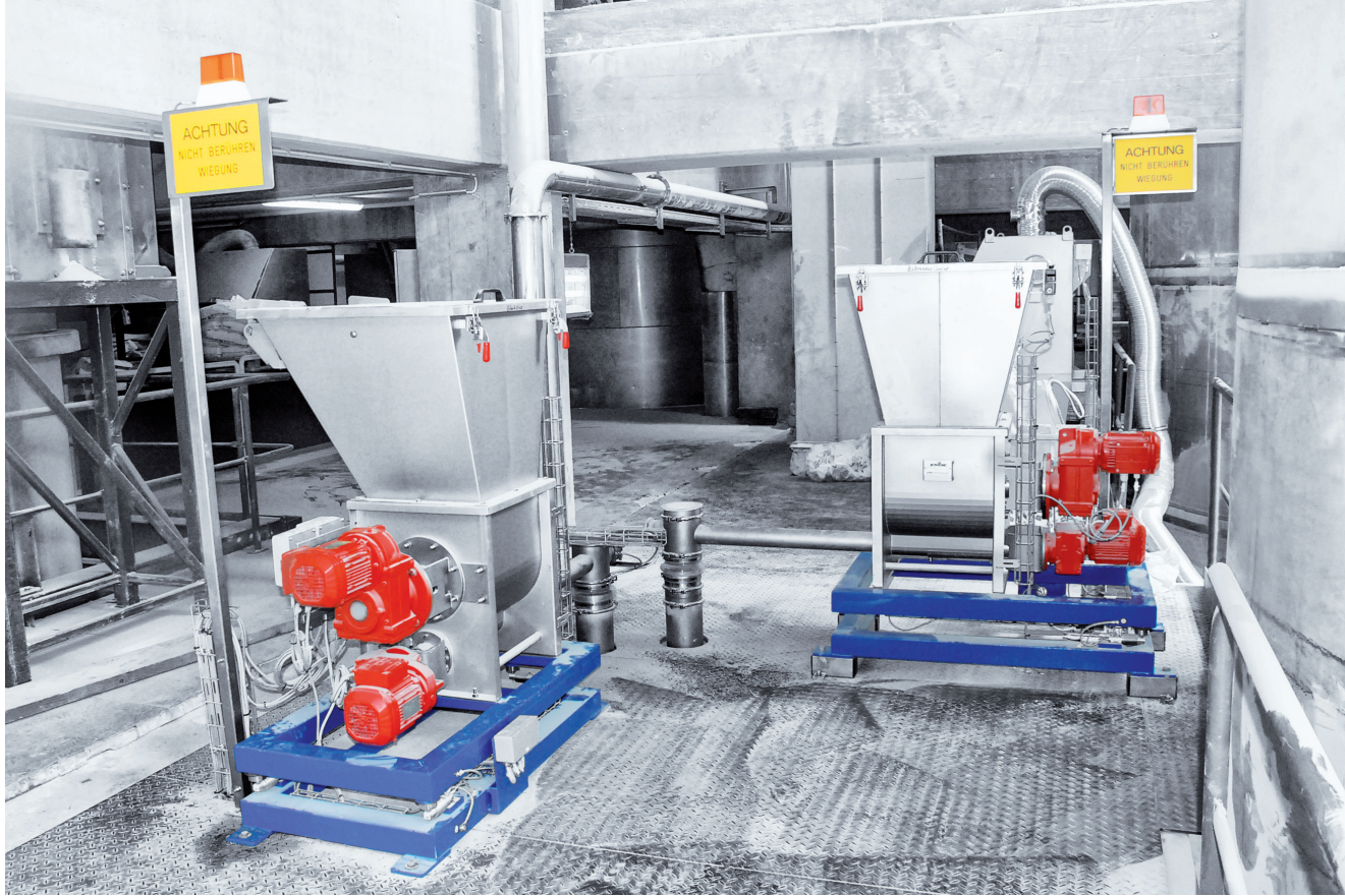
Batch dosing of additives in the salt industry
