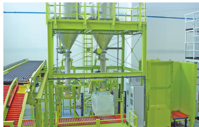
Double big bag filling plant for plastic granulate
