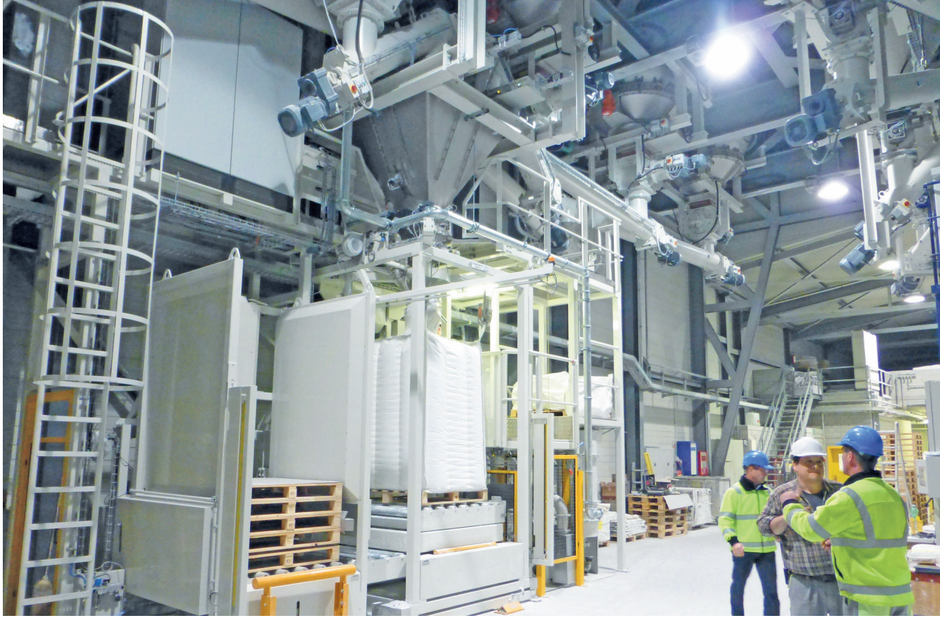
Big bag filling plant with pallet magazine and conveying technology for product out of onsite silos
