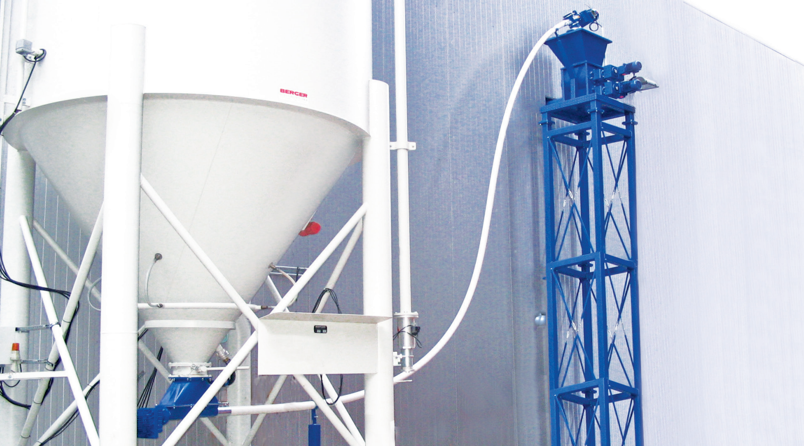
Silo discharge and metering screws - feed
